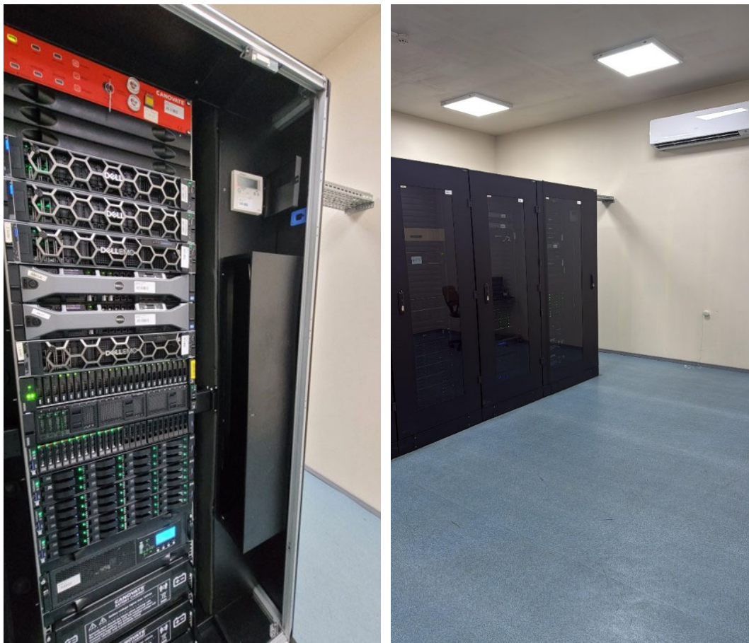
Figure 8.10. Physical layout of the server cabinets, in-row cooling and wall-mounted secondary cooling system.
