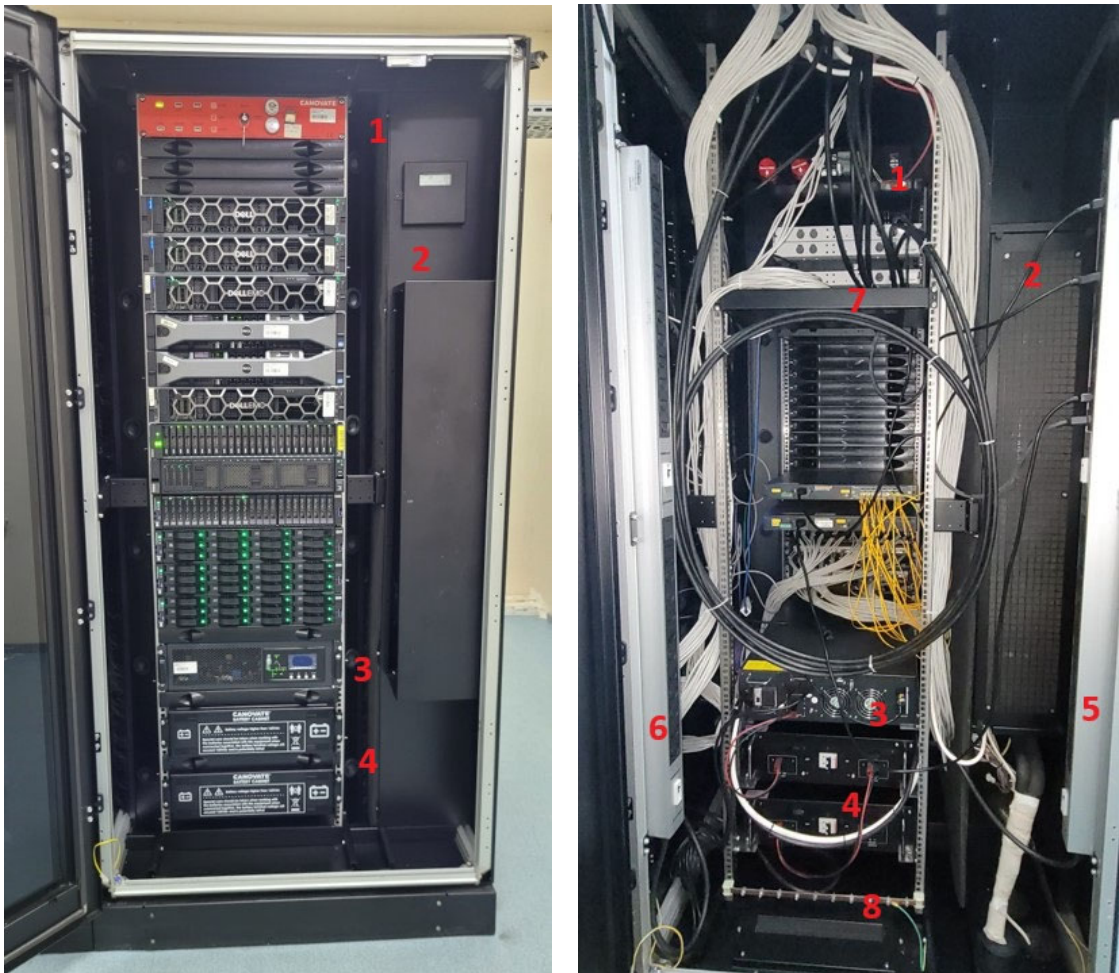
Figure 8.2. All-in-one rack cabinet front and rear view. (1. Automatic Fire Suppression, 2.IN-ROW Precision Air Conditioning, 3. Rack-Mounted Modular Online UPS, 4. UPS
