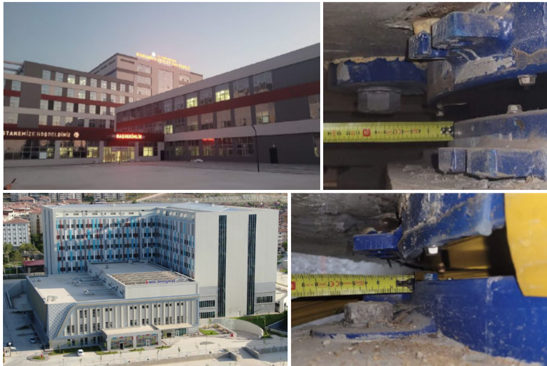
Figure 7. 2. Hospital buildings equipped with isolators and isolator statuses after the earthquake [60]
