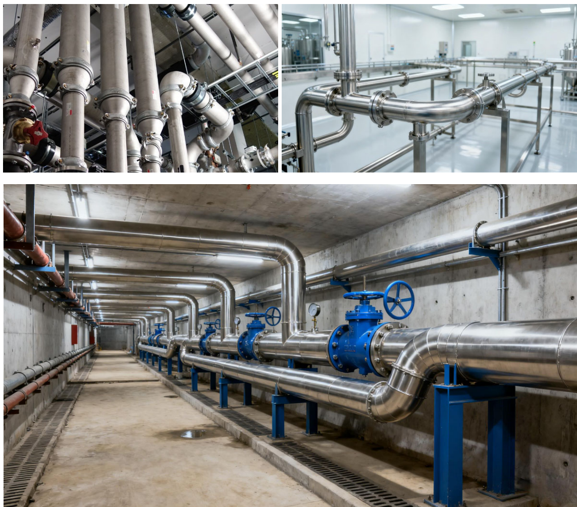
Figure 3.8 Stainless steel pipes in the healthcare facilities [37]
