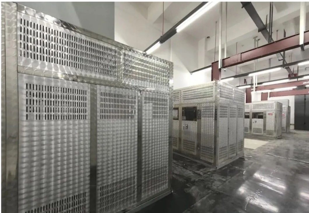
Figure 3.9 Stainless steel enclosures for power distribution [38]
