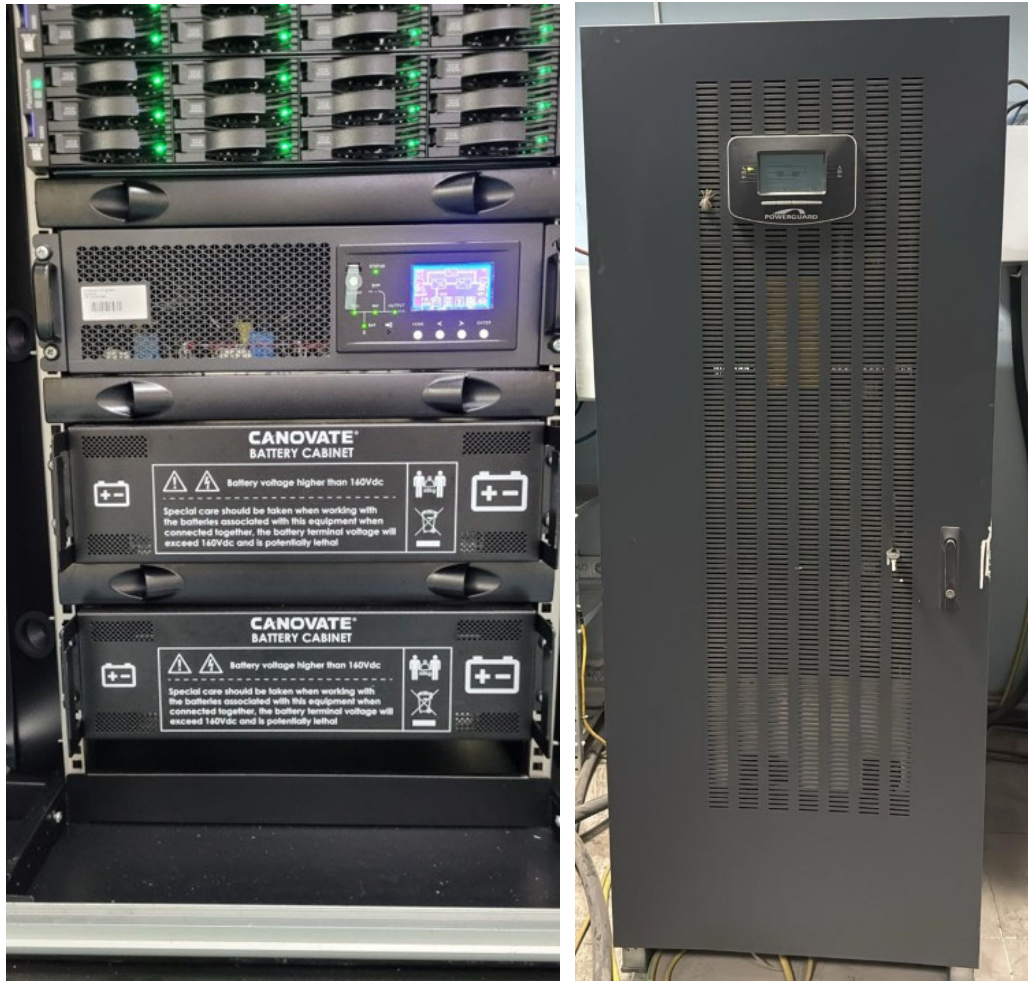
Figure 8.5. Rack mounted cabinet UPS and facility UPS used for data center
